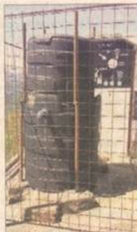
Biogas digester developed by JP University of IT, Wahnaghat.
